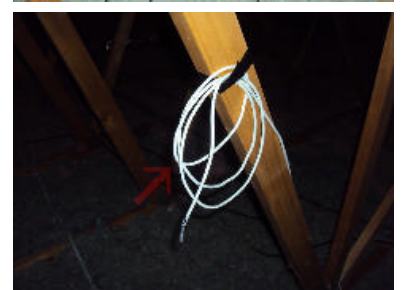
Image 3: Loose wires in different areas of the ceiling space, these are for hard wired smoke alarms that have not been installed.
