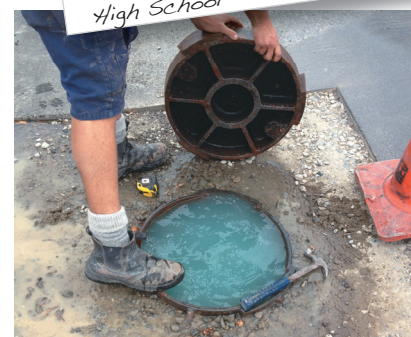
Hmmm - an interesting surprise when we lifted this storm water inspection hatch to find it full of sea water outside South Brighton Primary School.
